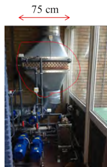
Figure 3.6: The installation of the tube-fin air cooler surrounded by a red circle. The two horizontal headers used to distribute the flow of hydrate slurry into 15 parallel circuits is clearly visible. Each vertical row of tubes is a different circuit.
